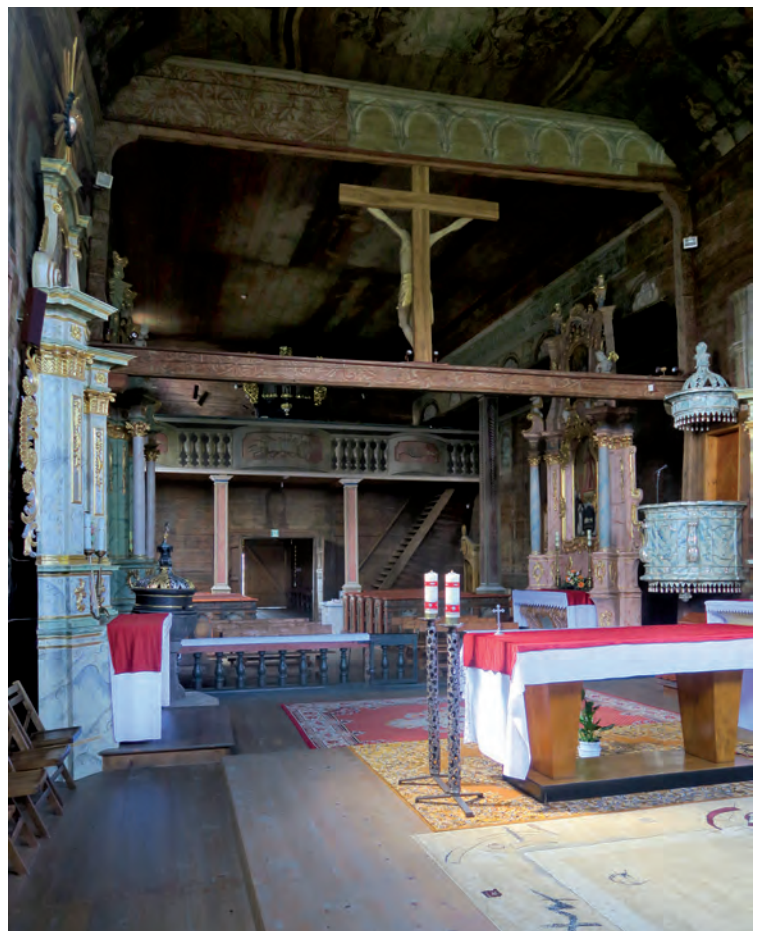
Church in Haczów – view of the rood wall from the presbytery side. Photo: M. Czuba
